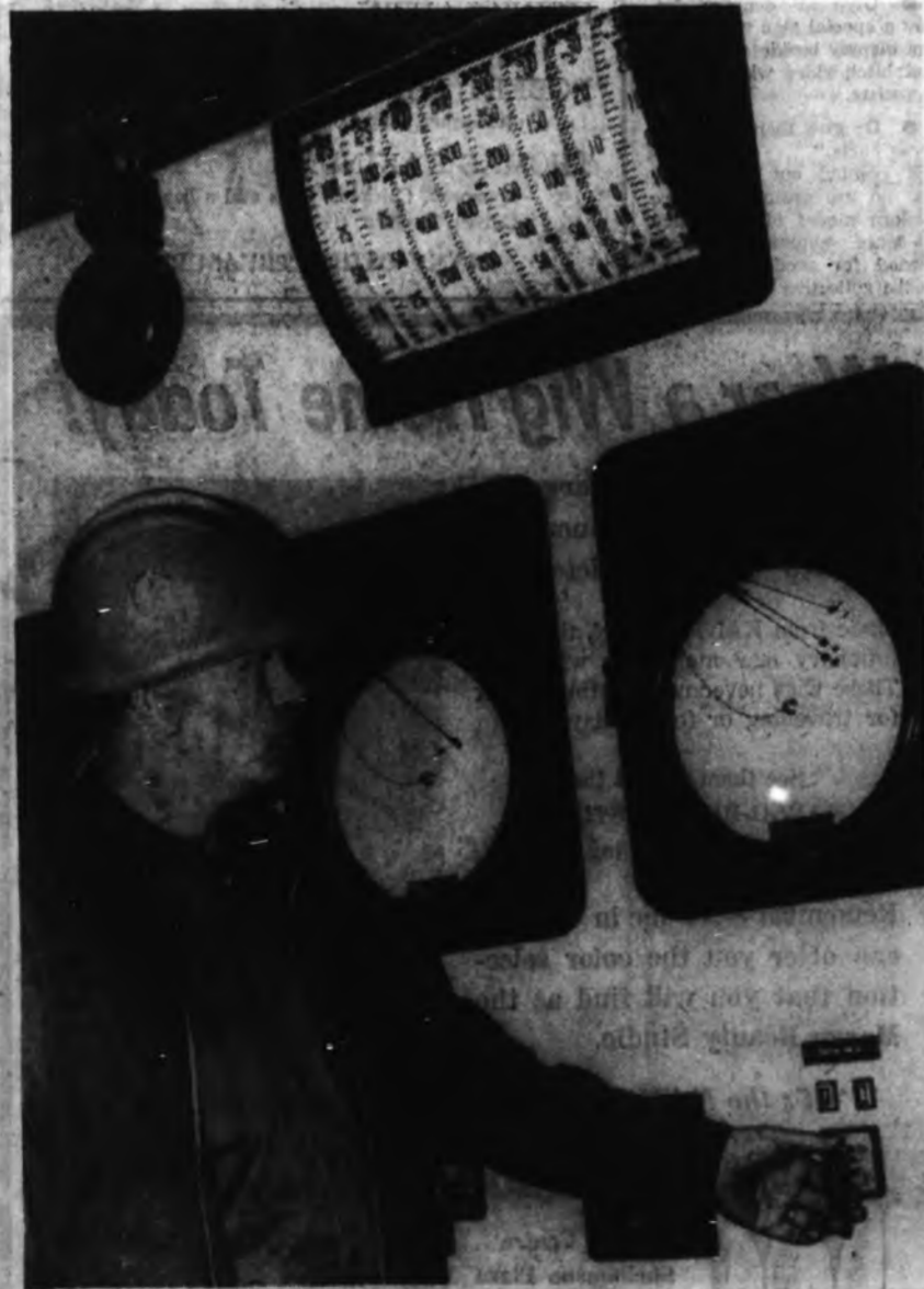
SETTING CONTROLS in powerhouse is Robert Burnside of Duncan. He is Youbou foreman and has
